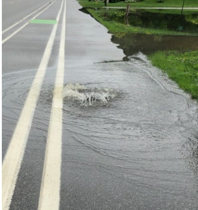
Old Tecumseh Road, Sanitary Manhole overflow of system surcharged, July 2021
