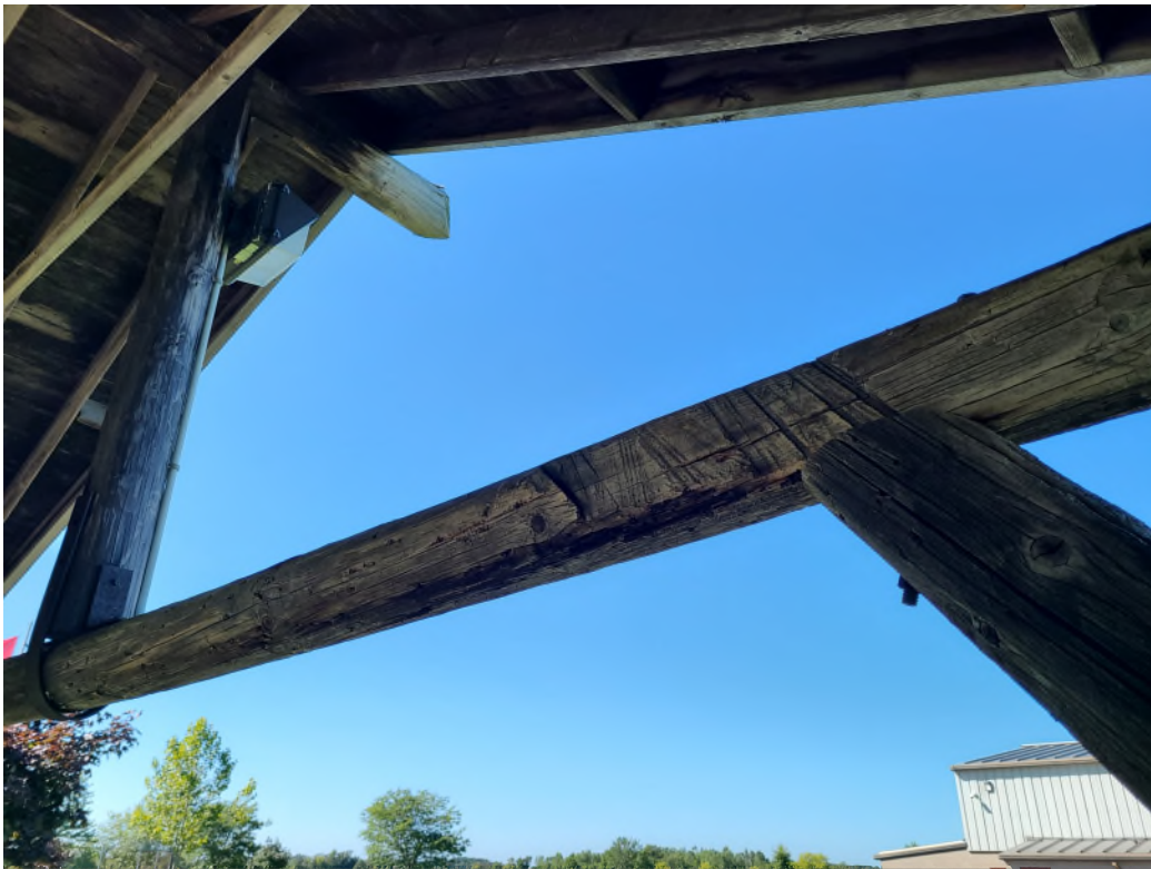
Photo #7: Significant notching, abrasion & checking on horizontal framing member
