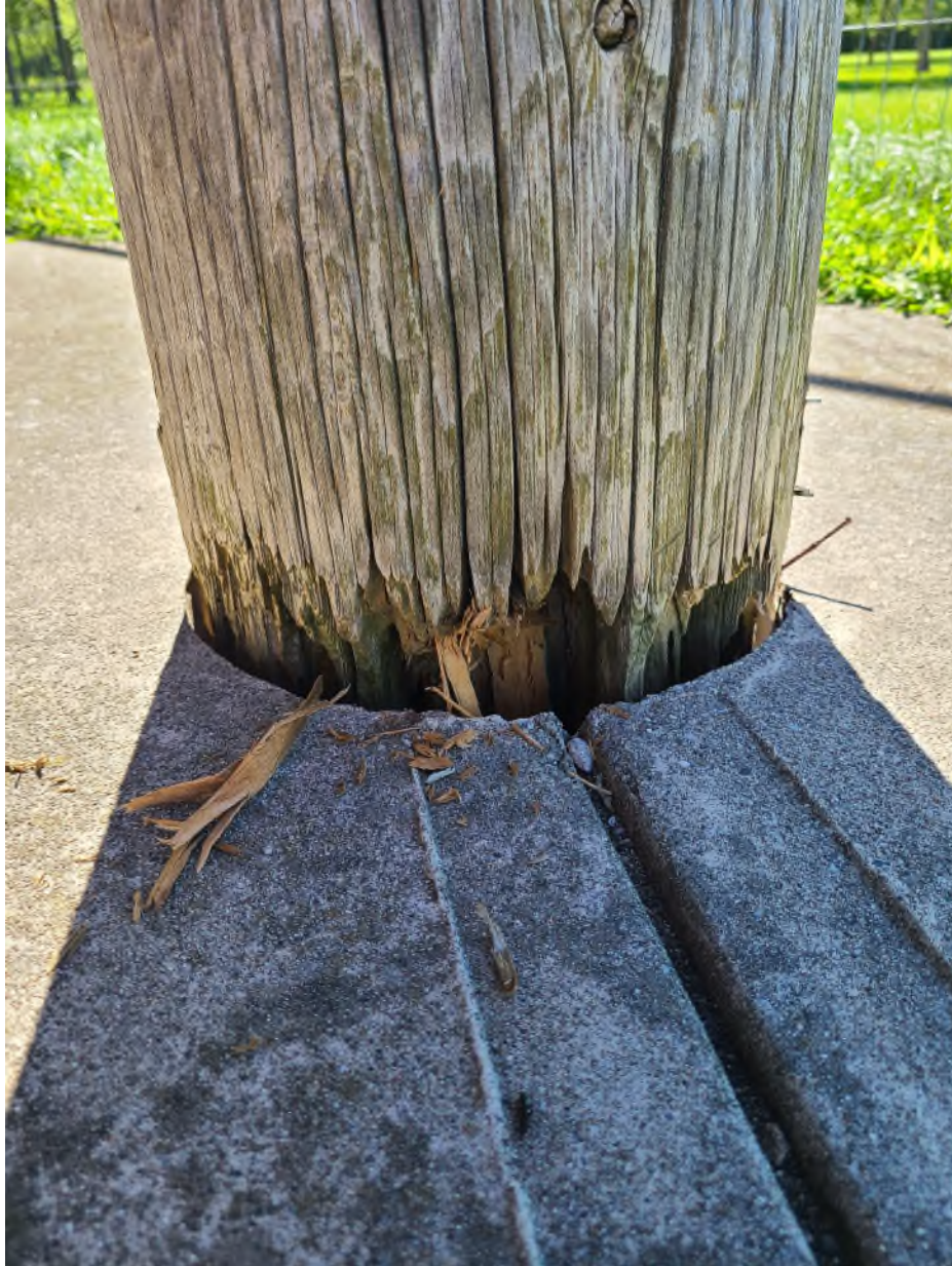
Photo #3: Substantial Timber Rot at base of Northwest Post Support
