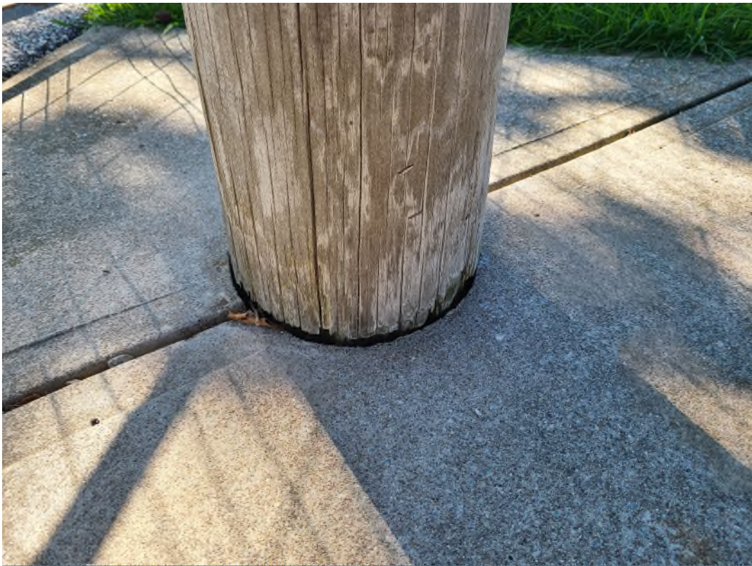
Photo #2: Timber Rot at base of Southwest Post Support
