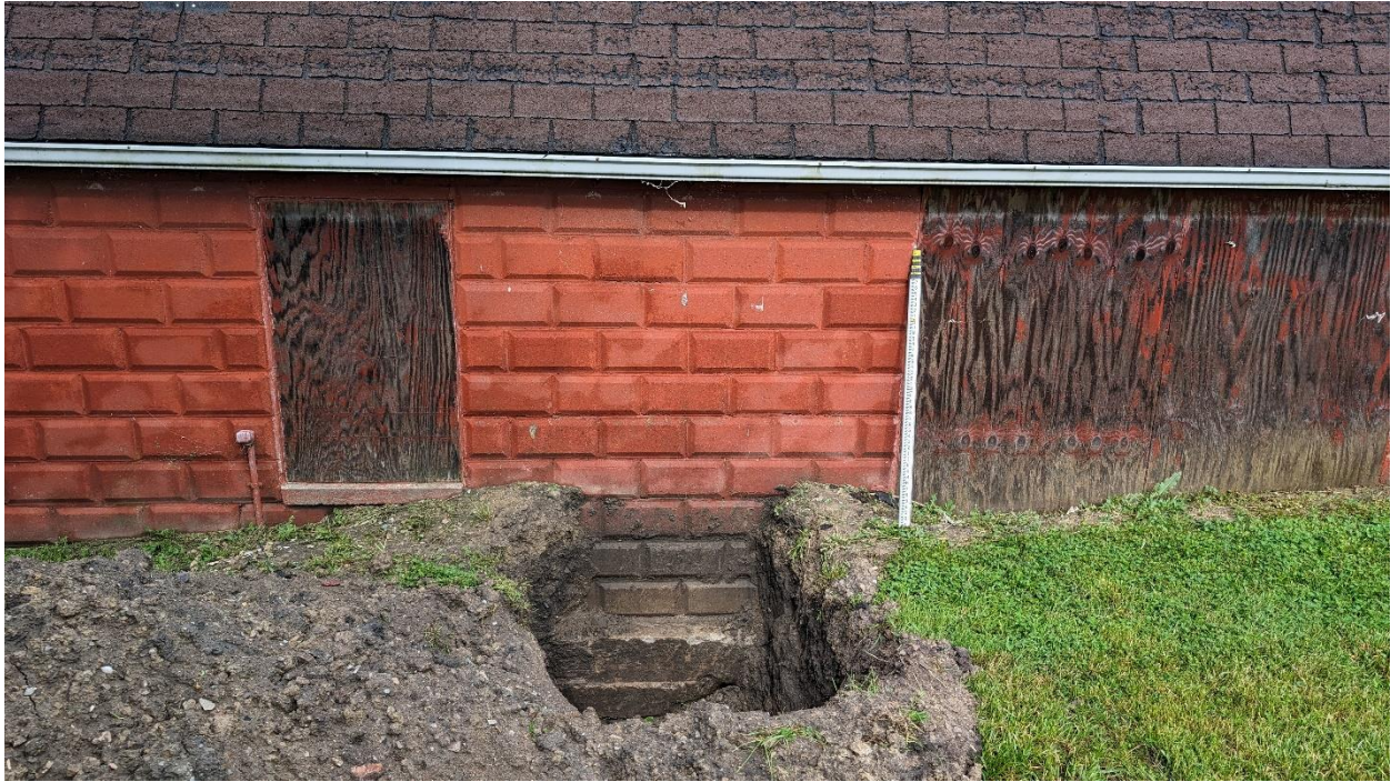
Figure 5 – Exposed foundation hole on the East side of the building (original portion).
