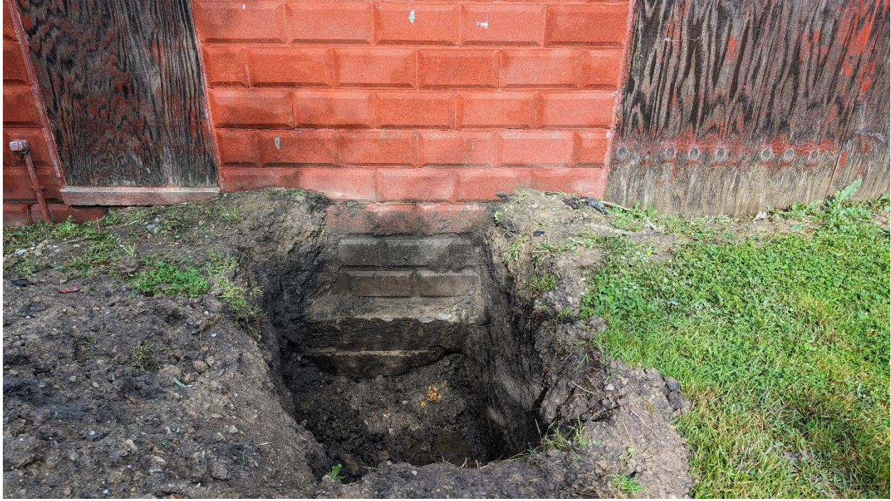
Figure 6 – Exposed footing on the East side of the original portion of the building.
