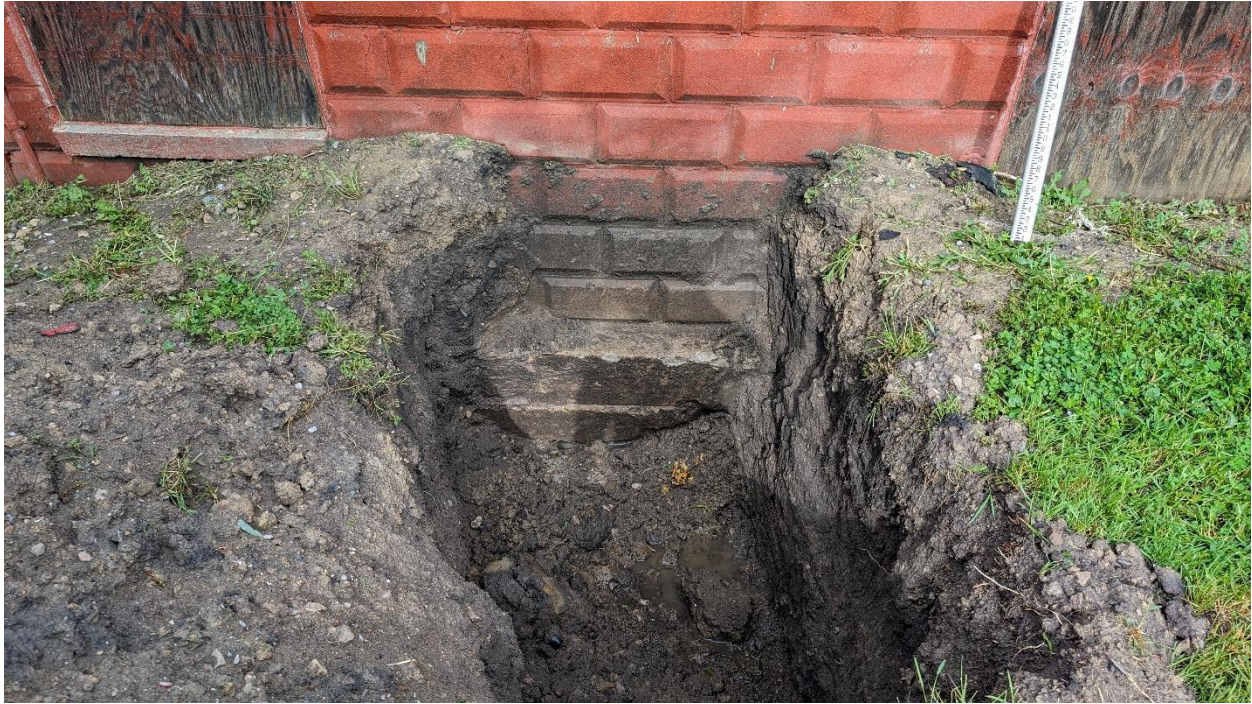
Figure 7 – Exposed footing on the East side of the building.
