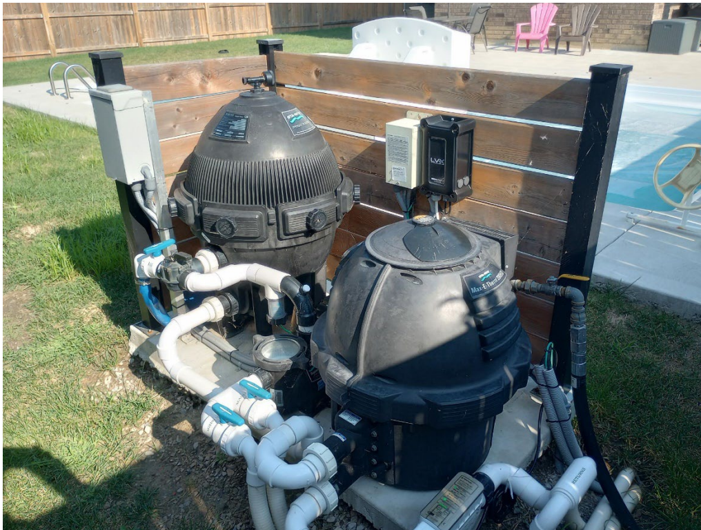
Figure 6: Existing pool equipment (to be moved) in southeast corner of lot.
