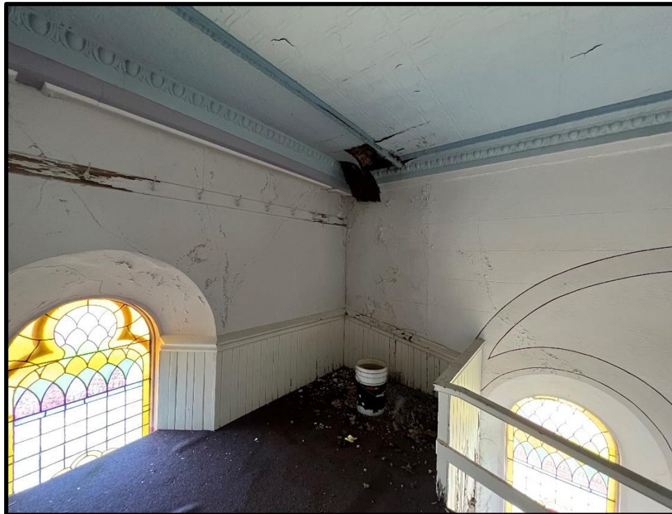
Image 42: 7119 Tecumseh Road Interior – Leakage Through Tin Roof in Balcony (Photo taken July 22, 2022)
