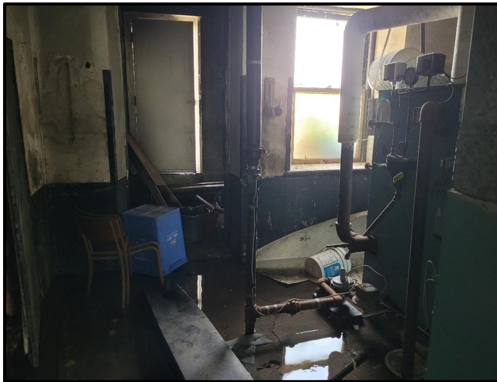
Image 50: 7119 Tecumseh Road Interior – Basement Mechanical Room (Photo taken July 22, 2022)
