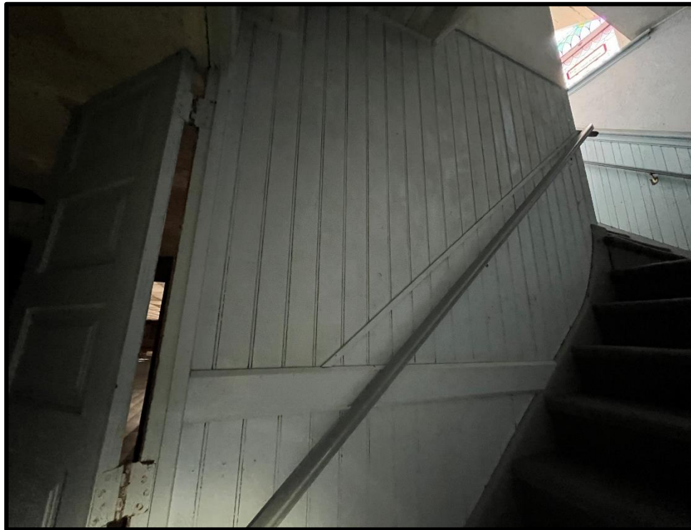
Image 44: 7119 Tecumseh Road Interior Detail – Beadboard Panelling in Basement Stairwell (Photo taken July 22, 2022)
