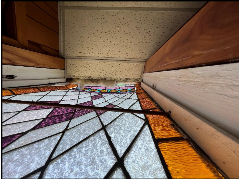
Image 57: 7119 Tecumseh Road Interior – Bowed and Warping Stained Glass Windows (Photo taken July 22, 2022)
