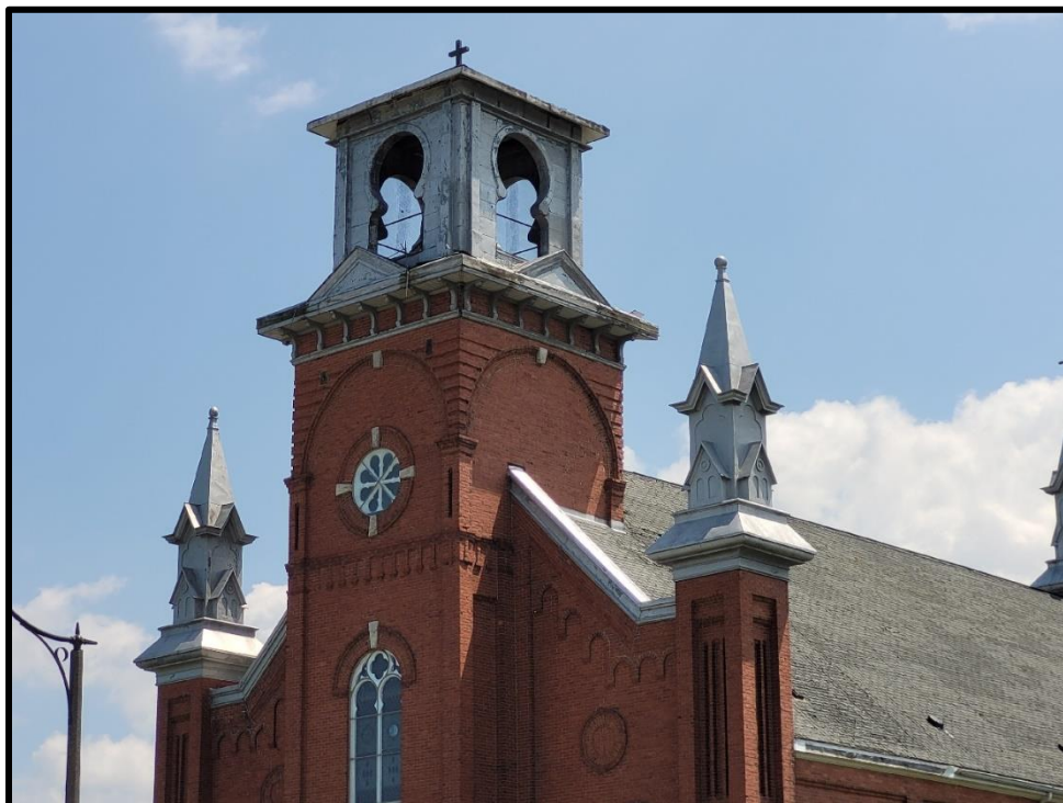
Image 10: 7119 Tecumseh Road Exterior – Pressed Tin Belfry, Parapet Walls and Pinnacles (Photo taken June 22, 2022; Facing Southeast)
