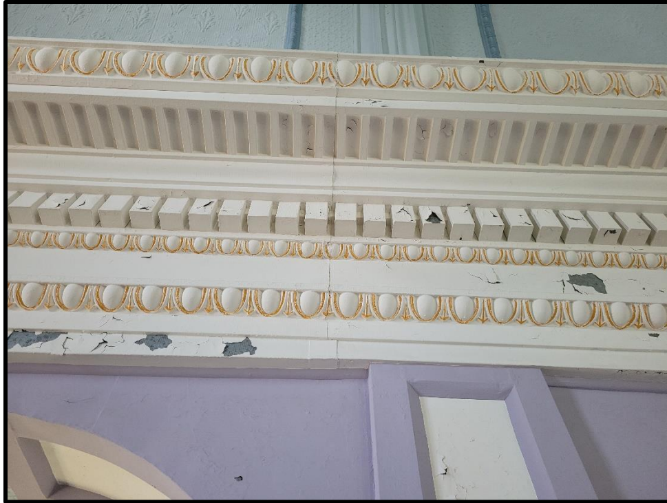
Image 29: 7119 Tecumseh Road Interior Detail – Pressed Tin Dentils and Egg and Dart Detailing (Photo taken July 22, 2022)
